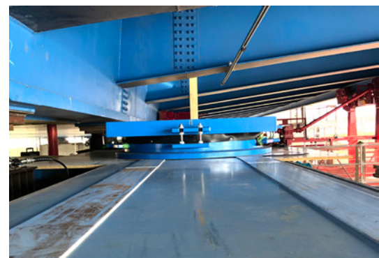
The new bearings were brought in place via a temporary launching track.
