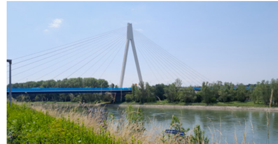
The Raiffeisen Bridge near Neuwied with the pylon on the Rhine island “Weißenthurmer Werth”.
