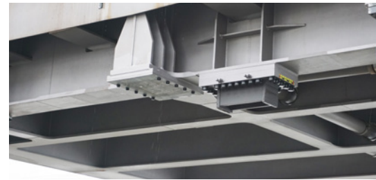
Bottom view of the opened new railway lift bridge; on the left the support surface for the multidirectional elastomer bearing, on the right the upper part for recoupling into the transversely fixed horizontal load bearing.
