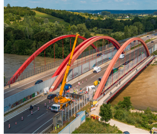
The Lech bridge near Gersthofen, west of Augsburg, with the construction site of the expansion joint replacement. The total replacement took just one weekend, with five hours of complete closure only.
