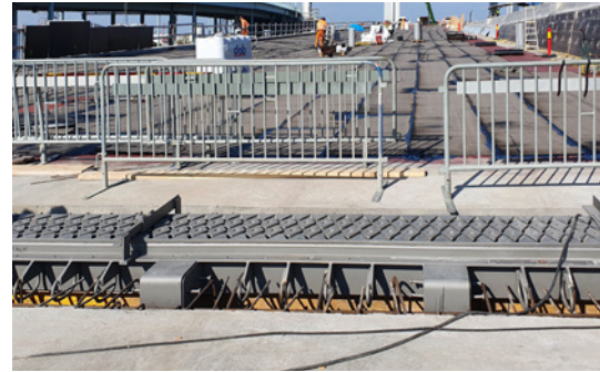
The expansion joint lifted into position with the lift bridge in the background. On the left: the former, higher bridge.
