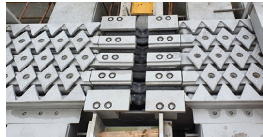
Track tunneling of the noise-reduced XL400 on the jobsite in Gothenburg: in the center the fitting pieces between which the track will be placed.
