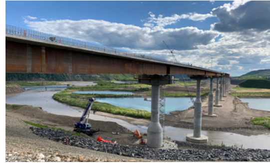
Halfway River Bridge under construction, May 2021. The tapered piers indicate the future water surface of the reservoir.
