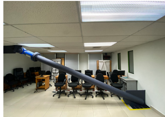
Built-in hydraulic damper: At the top with connection to the existing building structure ...
