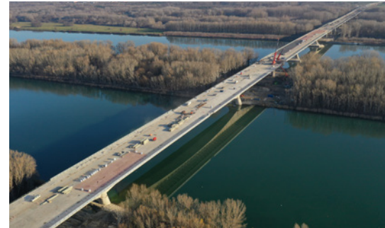
The fifth Danube Bridge for Bratislava features a length of about 3 km, and, besides the Danube, it also spans the Kayak and further branches.
