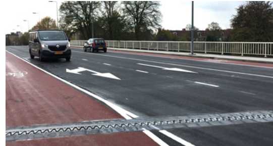
The new XC1, completely installed.
