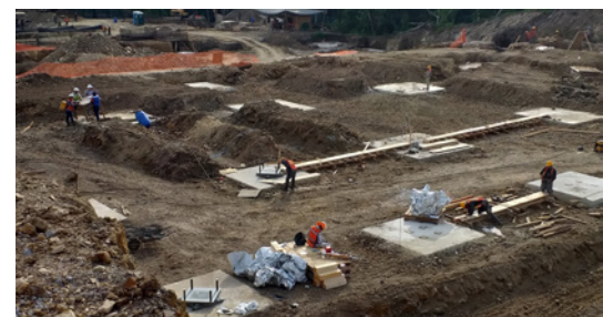
Construction site with foundations: seismic isolators are already positioned in the front and in the middle of the picture.
