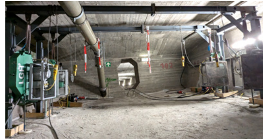
Electric winches in the bridge's box girder.
