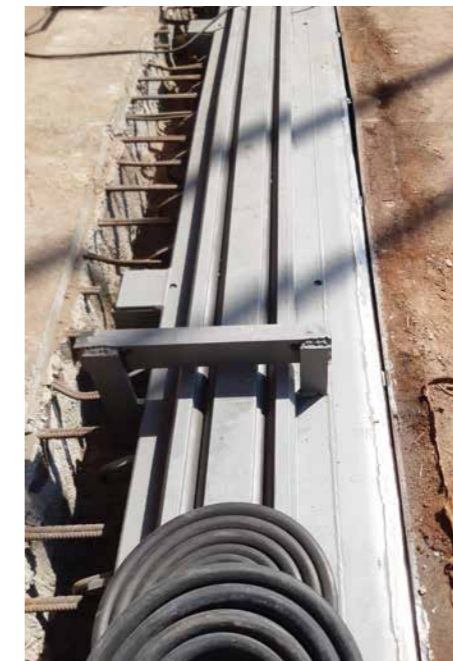
Installation of an expansion joint at the renovated bridge ends Photo: MAURER
