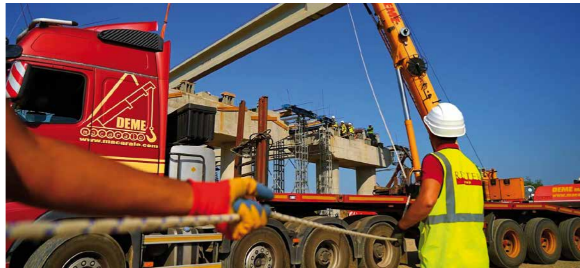
Sibiu-Pitesti motorway, several bridges with MAURER LRBs, SIP*s.
