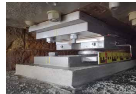
No more space was available: extremely tight spatial conditions at a bearing under a steel girder. Photo: MAURER
