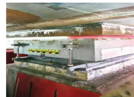
Bearing set in concrete prior to the lowering of the bridge. Photo: MAURER
