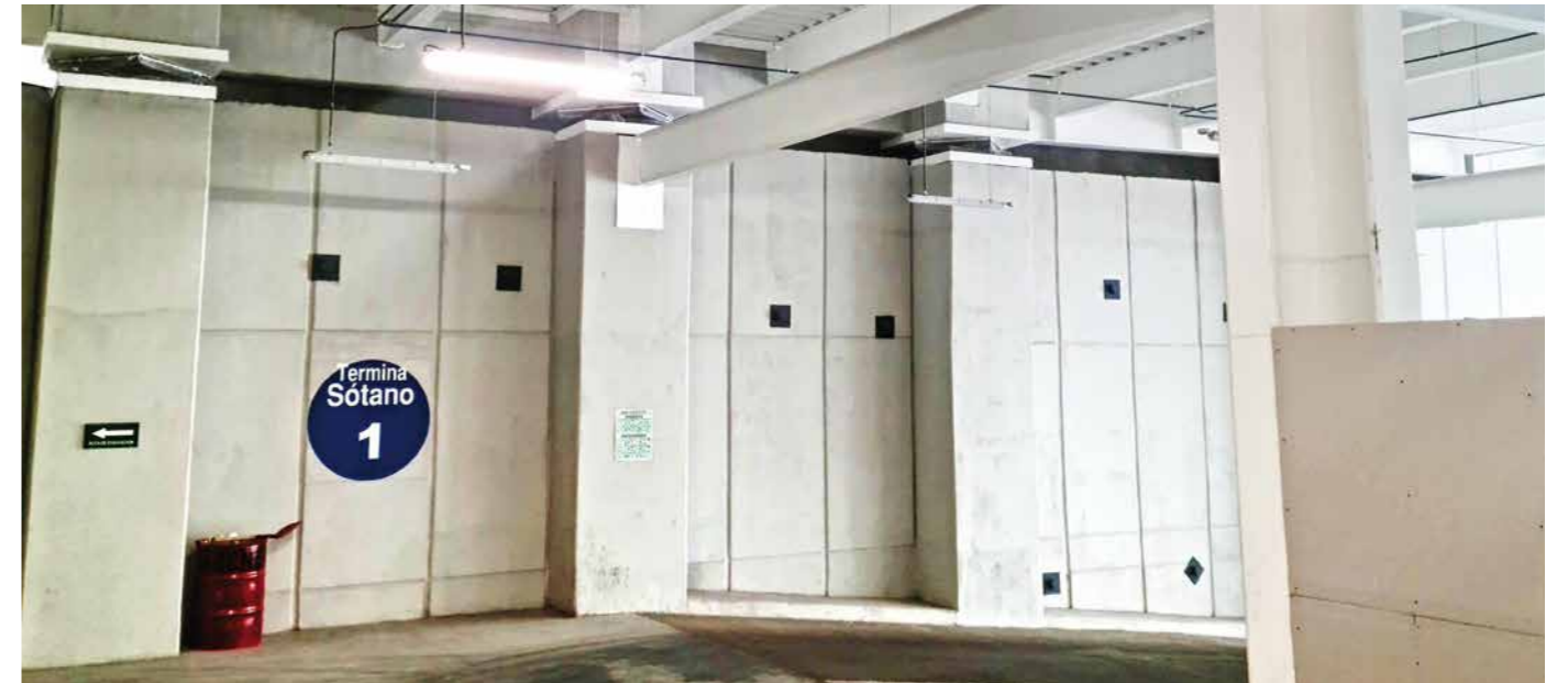
Four of the total 34 installed SIP®-A bearings on top of the support columns. Visible at the bottom is the descent to the underground car park. Photo: MAURER
