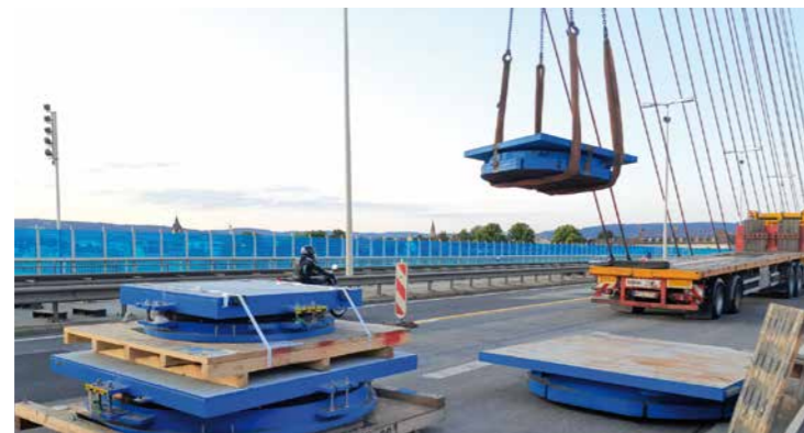
The new spherical bearings were replaced from the bridge deck. Photo: MAURER
