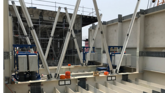
View of a bridge segment with four vibration dampers. They were manufactured entirely in Munich and then lifted into the box girder and fastened on site. The bridge segments are prefabricated on land.
