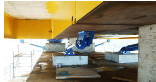
Situation on one of the two bridge pillars. Center front and on the right: two hydraulic dampers in transverse direction, behind them on the left one of four sliding isolation pendulums can be seen, behind that at the outside two longitudinal hydraulic dampers.
