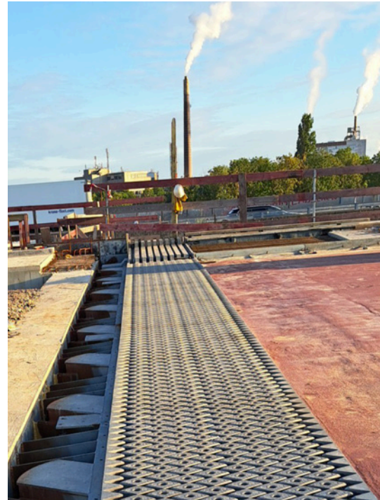
Detachable expansion joint: on the right, already integrated; on the left, still open – as here, the special detachable connection will be created and the lean concrete has not yet been installed.
