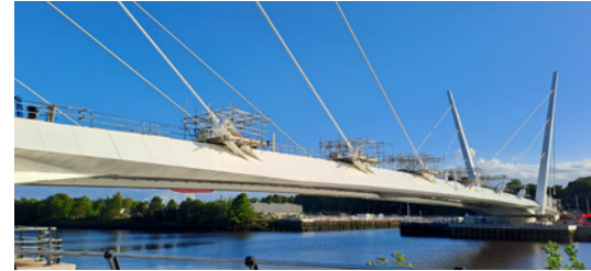
Even while under construction, the Clyde Crossing in Glasgow is an imposing and beautiful sight.
