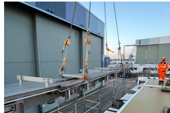
The expansion joint being installed at the pier in Rotterdam. The white section in the bottom foreground is the table on which the expansion joint rests, together with the dark sliding plates on which it slides.
