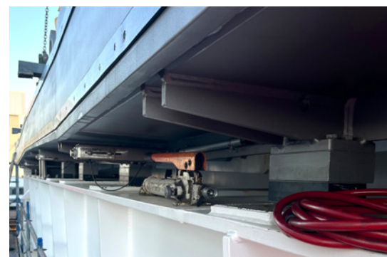
The installed expansion joint. When closed, it is only slightly wider than the white steel structure of the bridge. The two MSM® strips that absorb pressure when the bridge closes are visible at the top.
