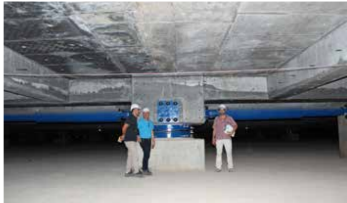
SIP Sliding Isolation Pendulum Bearing and two horizontally adaptive hydraulic dampers underneath the Mosque in Algiers. © KREBS + KIEFER Ingenieure GmbH
